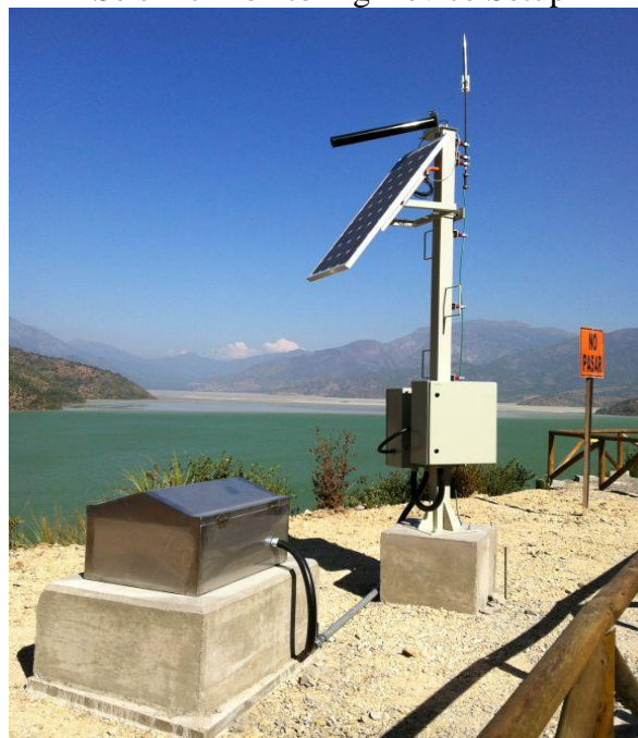
Earthquake seismic structural monitors
